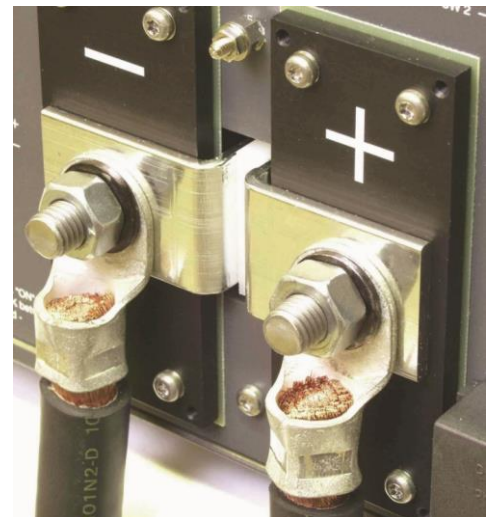
fig 5 - 1 Low resistive cable connection by mounting the cables directly on the DC output strips.
